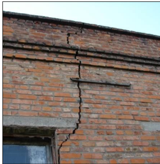
Fig. 1. A diagonal crack on a brick wall with a width ranging from 25 to 45 mm
